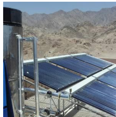
Fig. 2.6: Solar collecting panels on the roof.
